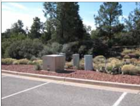
View of installed utilities.
