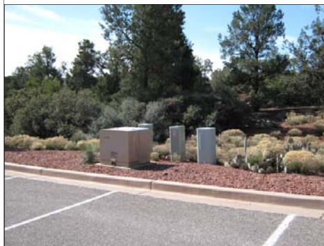
View of installed utilities.
